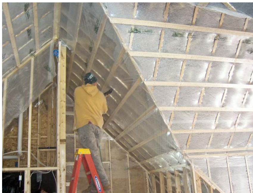
Figure 9. Triple-ply Par/Pac membrane is stretched around framing edges and rigorously stapled to prevent the cellulose insulation from bulging past the wall plane. Cellulose is blown through slits in the membrane to a density of 3.5 pounds per cubic foot. The slits are then resealed with tape.
