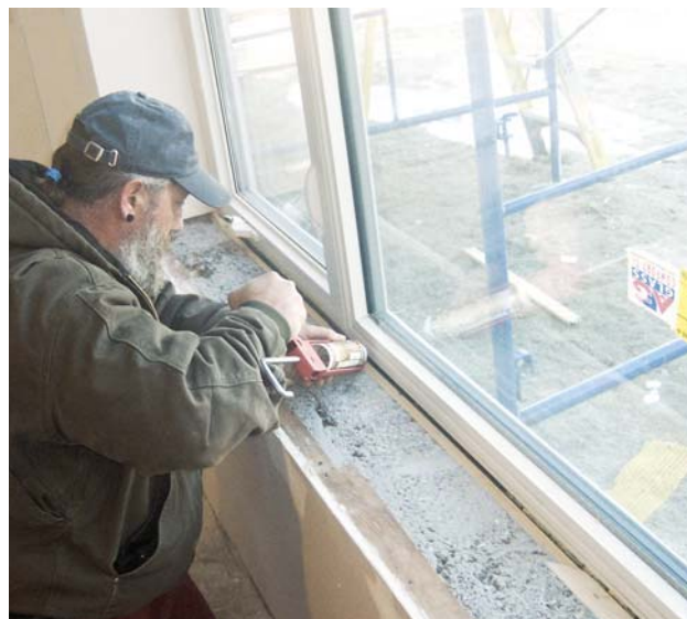
Figure 11. Condensation on a very cold day during construction indicated gaps around this window that were not revealed during blower-door testing. The author stripped back the dry-wall returns and caulked around the jambs.
