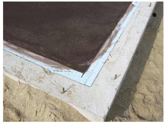
Figure 1. Four-inch-thick foam board provides R-20 insulation under and around the edges of the radiant floor slab (left), which is tinted chocolate brown to serve as the finished floor. The inside 2x4 wall of the 1 1 / 4 -inch-thick double framing will cover the exposed foam around the perimeter (above).
